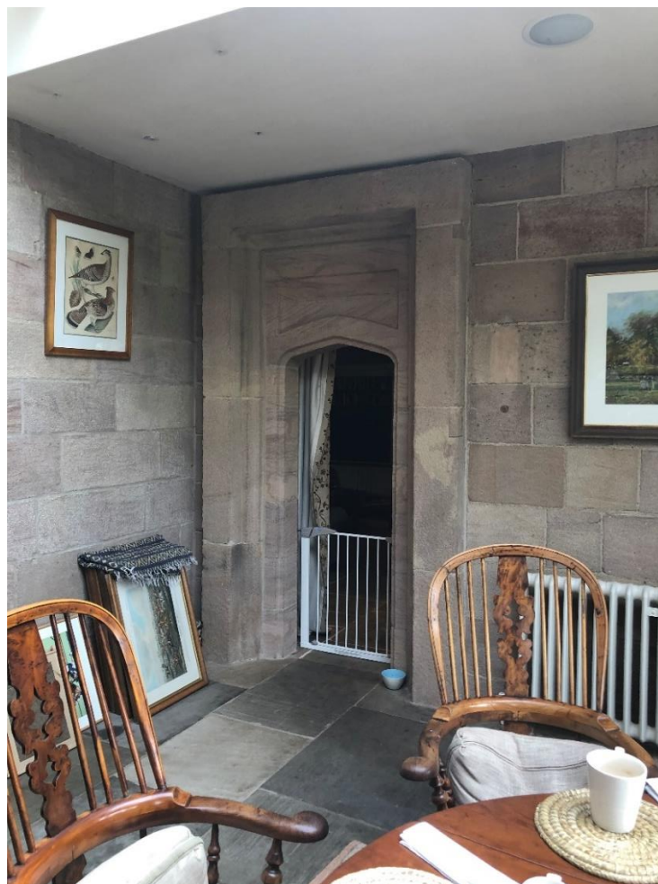
Fig.14: re-set 19 th century doorway between the orangery and the 1990s east wing, from the west (Seven Architecture)
