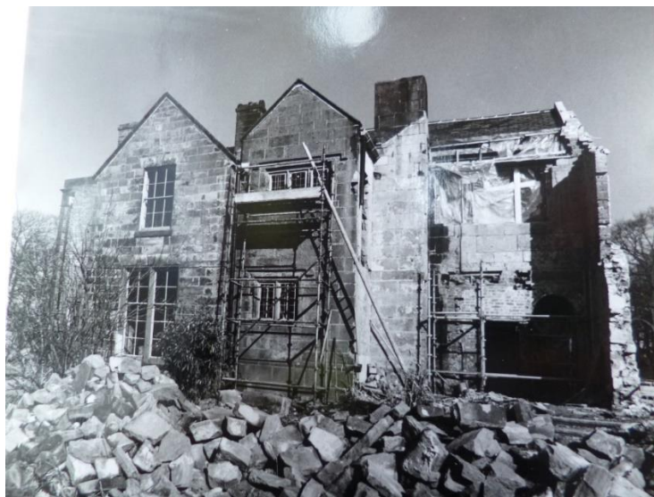
Figure 5: south elevation after clearance of Victorian east buildings, early 1980s (client collection)
