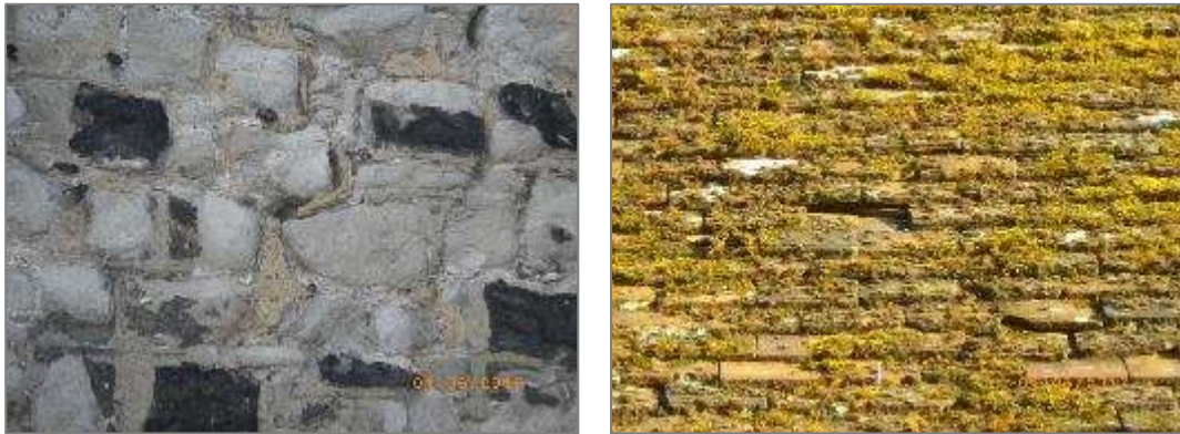
Cavities within external masonry and missing roof tiles on the northern roof pitch of the nave
