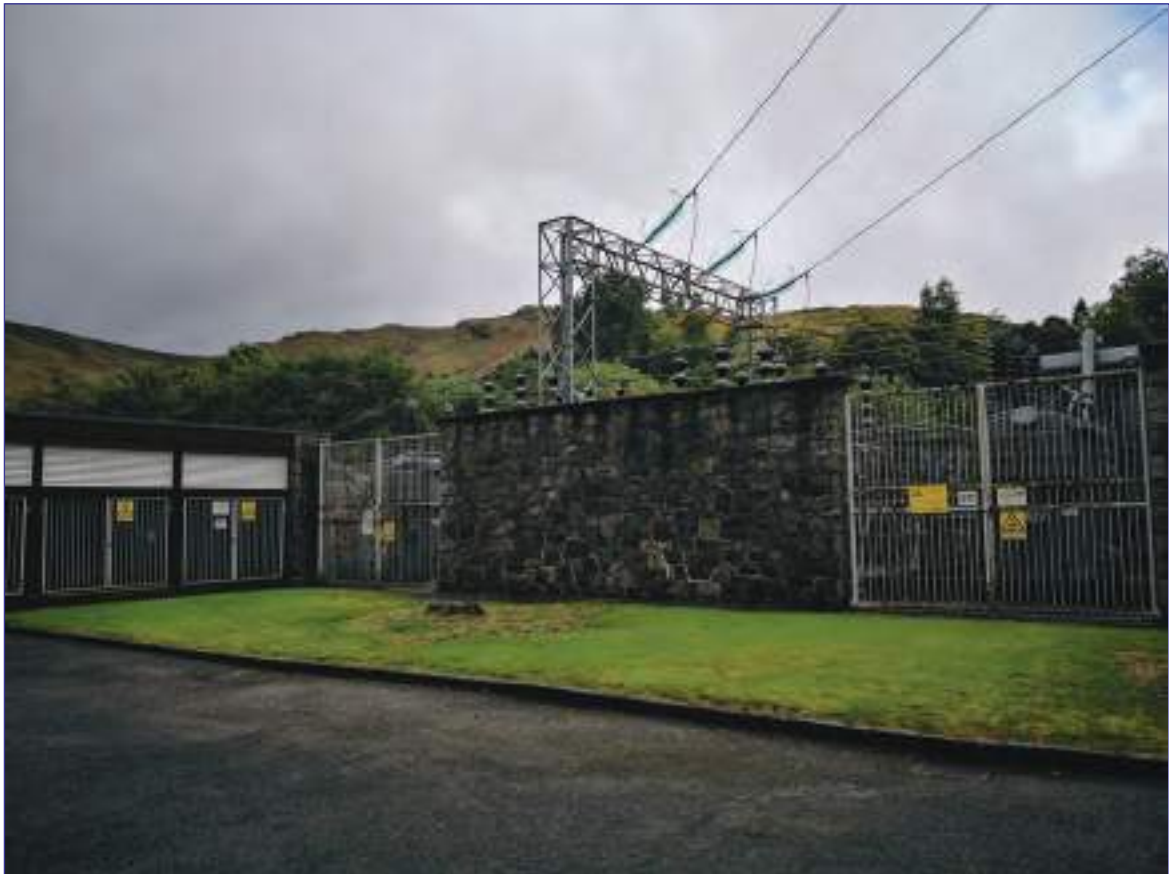
Plate 1: West facing view of existing substation (Option 1)
