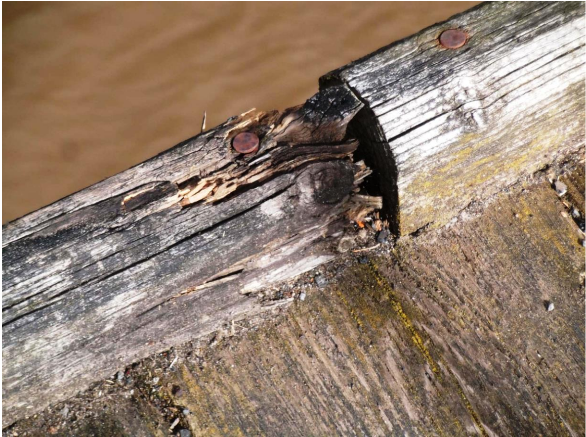
2018 DECAY & DAMAGE TO TOEBOARDS
