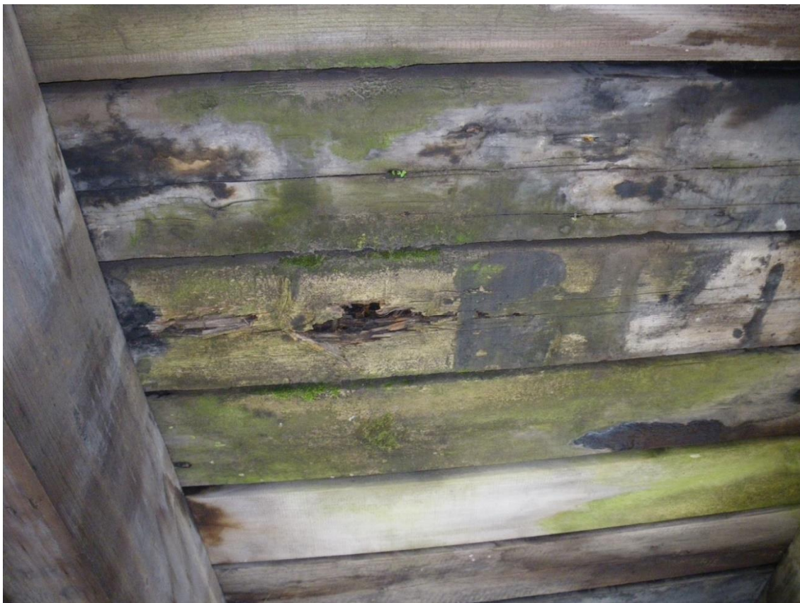
2018 DECAY TO LONGITUDINAL TIMBERS
