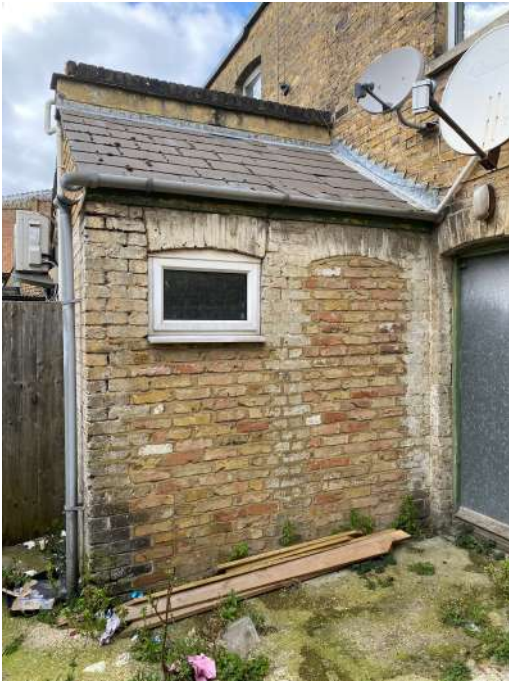
Plates 2 - Rear ground floor toilet area, where we are proposing a new ground floor extension
