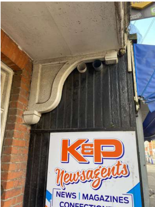
Plates 4 -Purpose made joinery and mouldings will be replicated on the new proposed shop front
