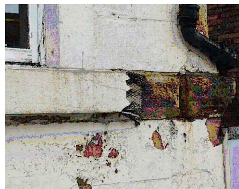
Photo 2 - 3rd floor End cornice condition (Example of render condition)
