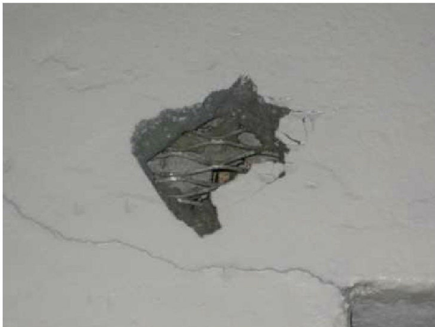
Evidence of Galvanised Mesh
