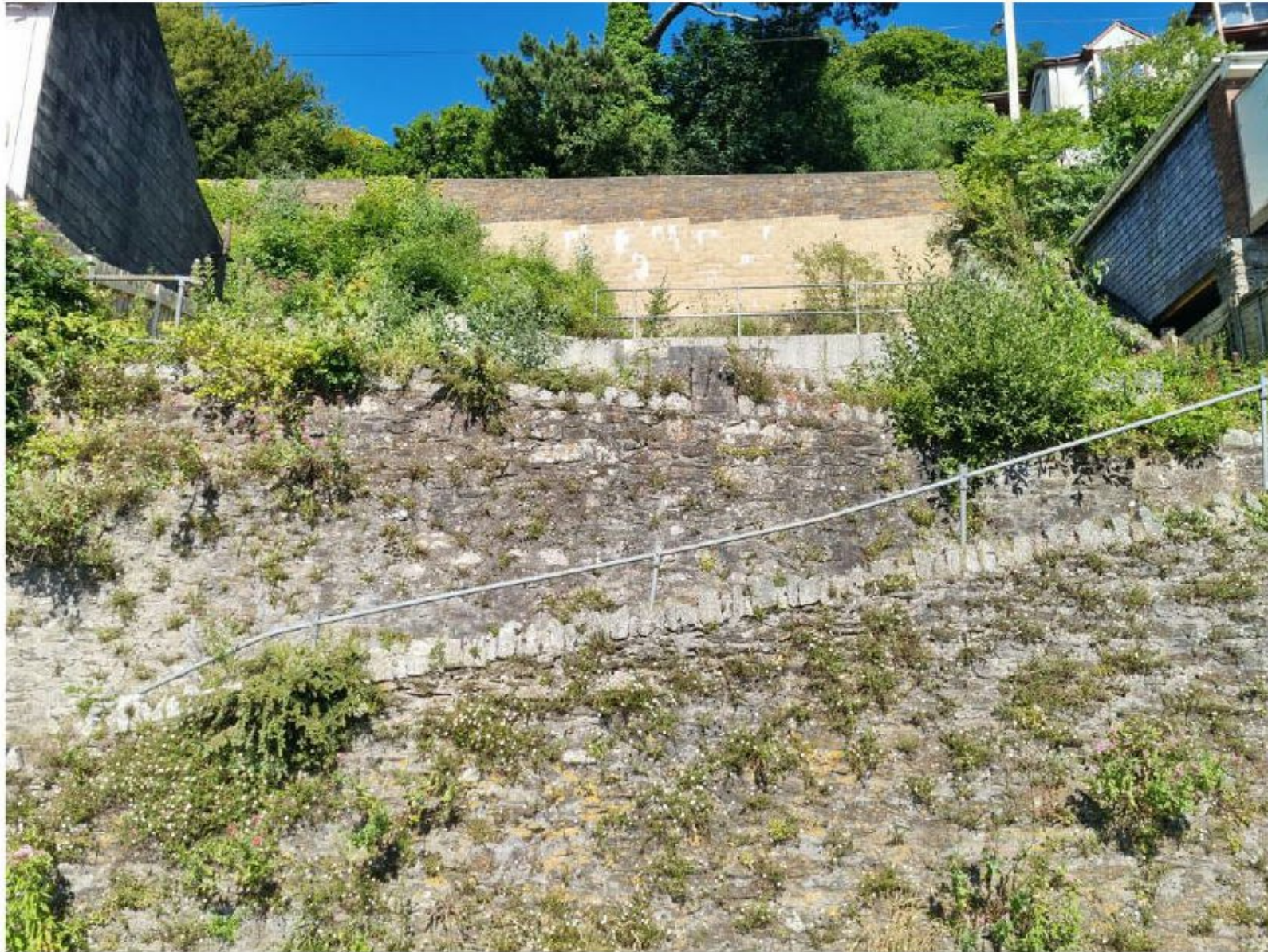
Figure 1 - Vegetation on stone facing walls.
