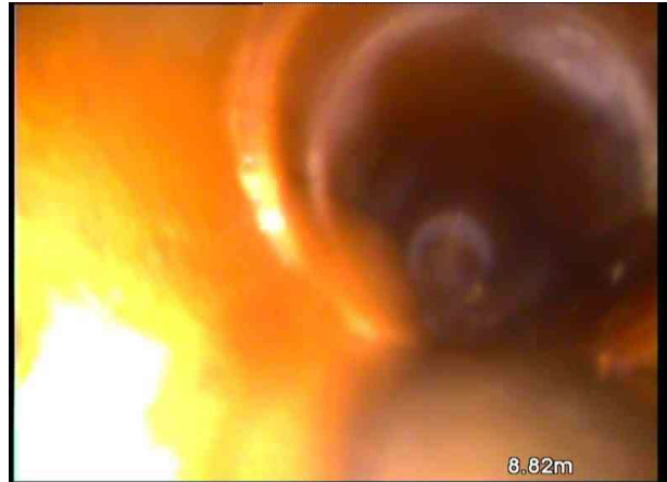
R_EX_6c2bc7a6-4ca9-4381-b2d8-ce4bed2d4871_20210831_114126_080.jpg, 00:03:31, 8.82 m Crack, circumferential at joint from 12 o'clock to 12 o'clock
