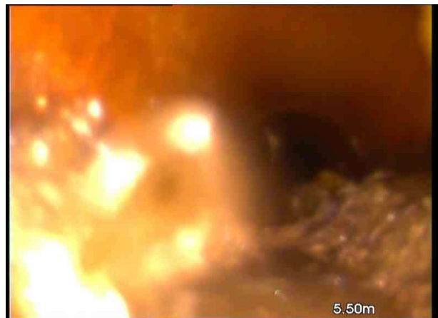
R_EX_d1903cee-7226-4cd5-aa22-3e67f3164058_20210831_113935_789.jpg, 00:02:42, 5.50 m Roots, mass, 45% cross-sectional area loss
