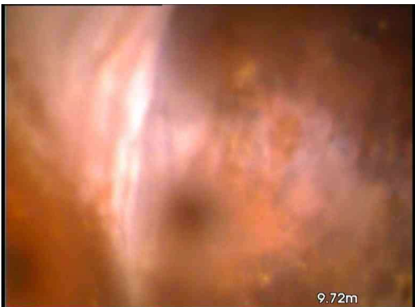
R_EX_d25a7815-0dd3-4ef0-8883-73cade75bfce_20210831_14237_000.jpg, 00:03:44, 9.69 m Finish node type, manhole, reference number: Main run, Back drop
