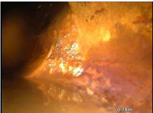
R_EX_46738934-6b8e-42d2-a93a-416dd35a5a63_20210831_1 113531_487.jpg, 00:00:44, 0.78 m Water level, 5% of the vertical dimension
