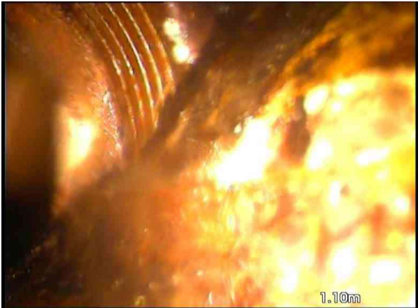
R_EX_da87cf2a-4cd9-4542-adf4-8fe13c085c4c_20210831_113647_577.jpg, 00:00:52, 1.10 m General photograph taken at this point, Buried manhole with connection
