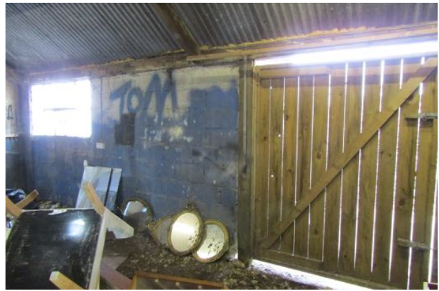
Plate 6. Gaps above doors
