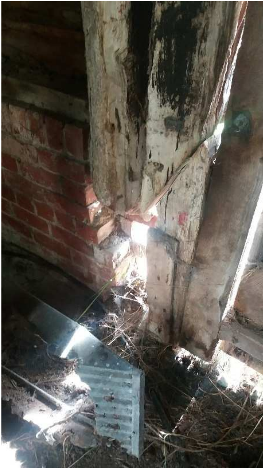
TYPICAL PHOTO WHERE SUPPORT LOST AT POST BASE
