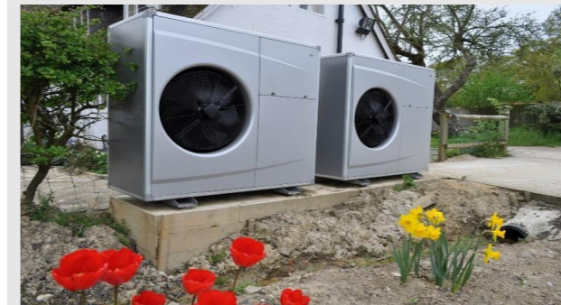
Outdoor units of an ASHP system (discharge)
