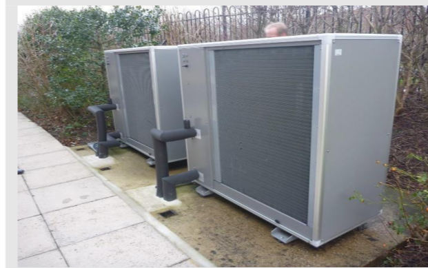
Outdoor units of an ASHP system (intake).
