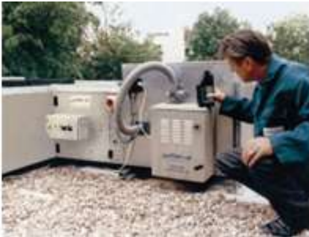
Figure 16: Example of an odour neutralising unit
