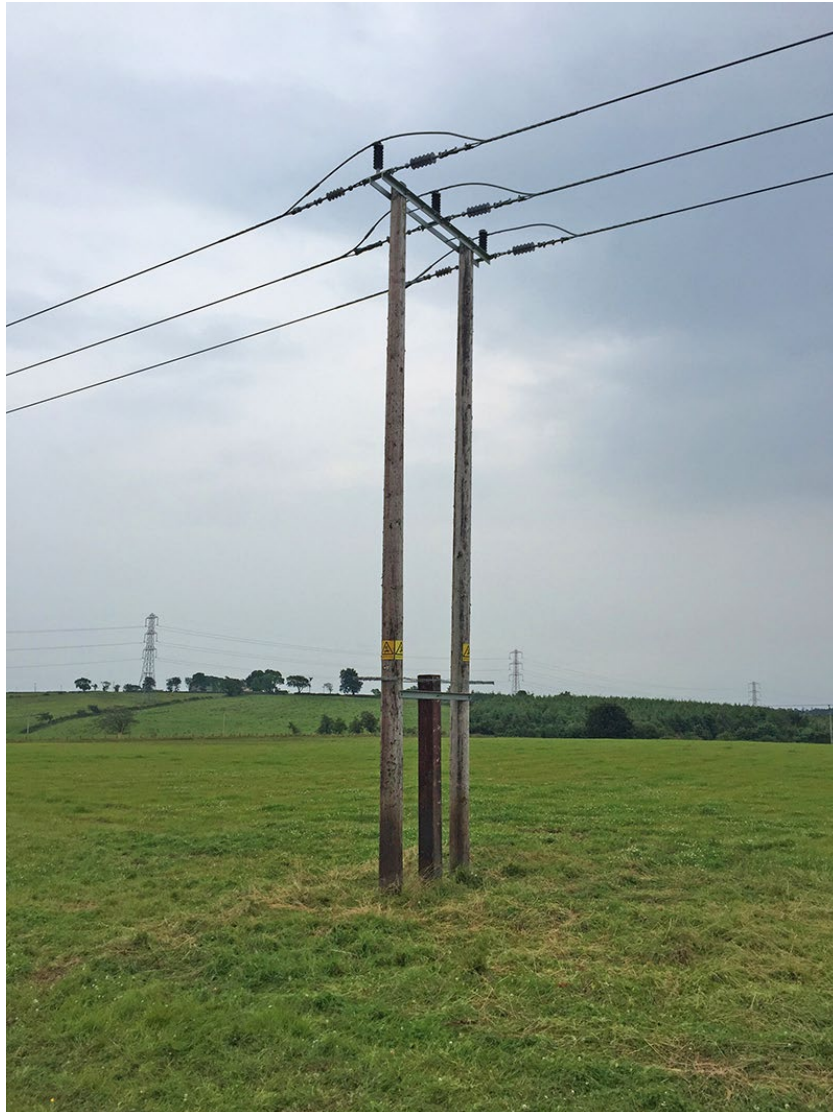
Photo 4.1: Typical 33kV Wood Pole – double or 'H-pole'
