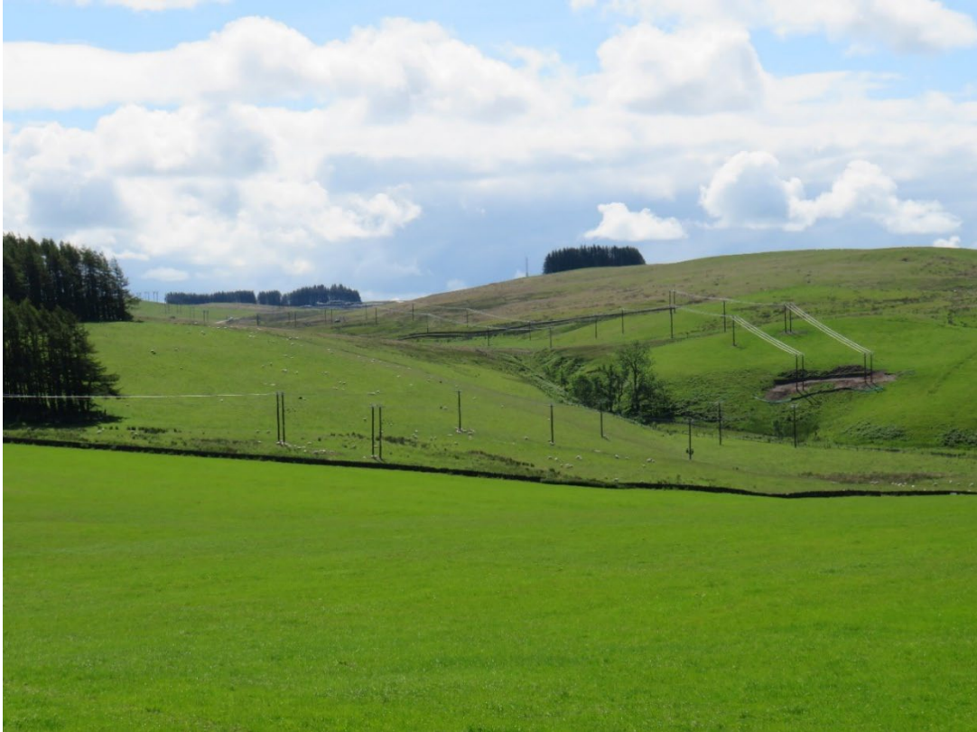
Photo 4.2: Typical twin 33kV Wood Pole Overhead Line
