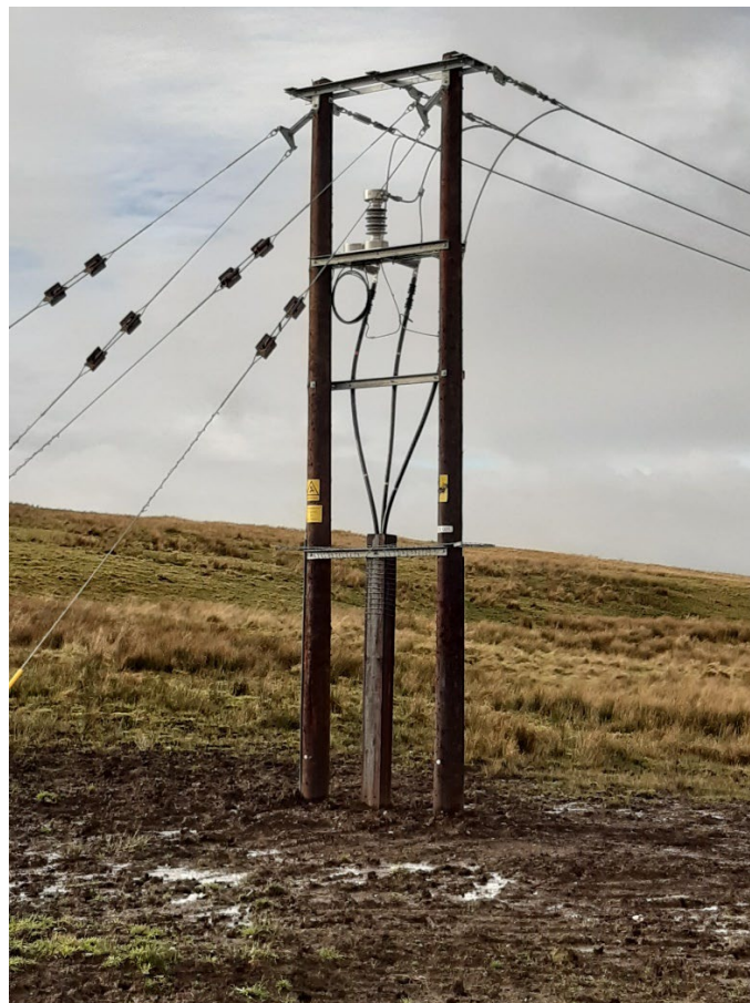
Photo 4.3: Typical Terminal Structure for a Wood Pole Overhead Line
