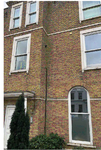
SAMPLE OF BOILER FLUE as at BUILDING on OPPOSITE SIDE of ROAD
