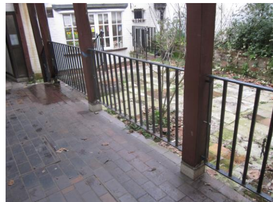
7. The railings that are proposed to be replaced. The timber supports to the canopy will be removed.
